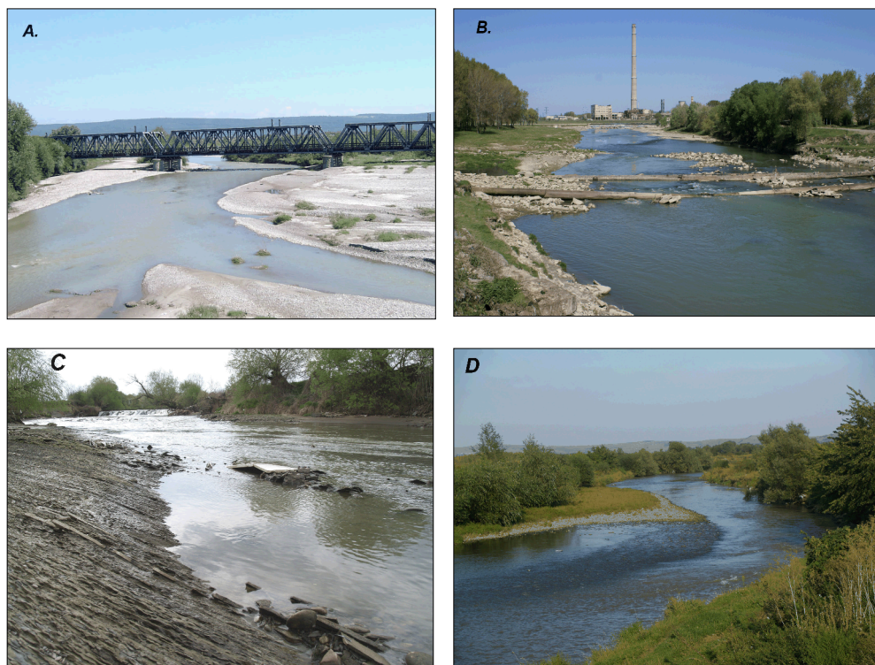
Fig. 11. Illustration on the river bed behaviour at the certain fluvial processes: aggradation, Trotus River at Adjud (piers are buried in 3 m of sediments)(A); degradation, Suceava River at Suceava (transversal pipes were initially buried at 2 m in the sediment, and today, after 20 years, these are digged out)(B); degradation, Somesu Mic River downstream Cluj Napoca, where the bedrock is uncovered (C); erosion and accumulation in balance, Somesu Mic at Someseni (D) (foto N. Rădoane, A. Perșoiu).
